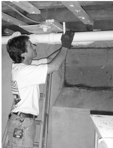
Joe Farringer, Schofield Plumbing, Freeport, works on new plumbing in 1889 school basement.
