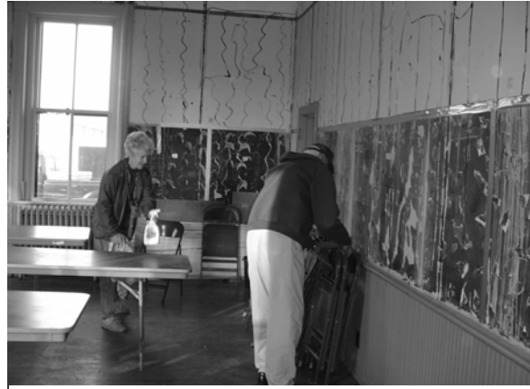
Judy and Harlan Corrie helped prepare the first floor of the 1889 school for the appearance of the contractor who will install the heating and cooling system starting the first week of November.
