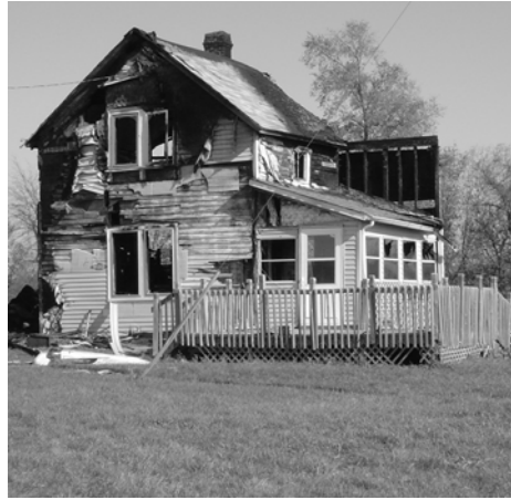
The house on West Cedarville Road was gutted by fire in 2008. This is how it looks today.
