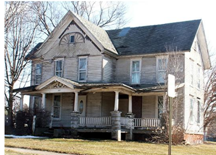
2014 photo showing collapsing front porch
