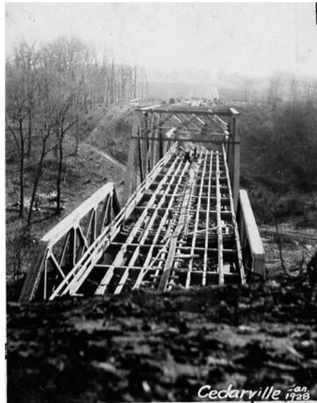
Construction of 1927 bridge over Cedar Creek. Black and white photo taken by Merton M. Memler, engineer in charge.
