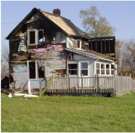
The house on West Cedarville Road was gutted by fire in 2008. It was later torn down and a new house constructed.
