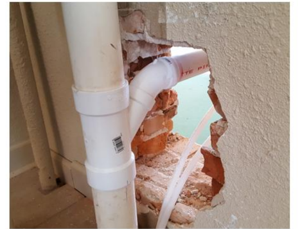
Drain and water lines connection to vent in second floor research library. Electric lines will follow the path of the water lines. All construction will be boxed and hidden from view.
